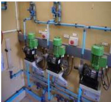
Neat chemical dosing room with backup dosing pumps
