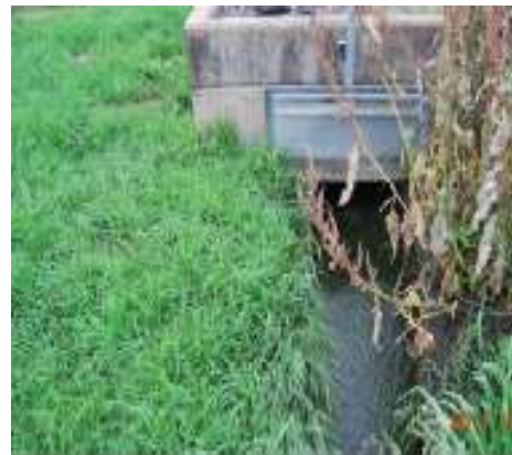
Overgrown sludge dam: sludge currently sent to river
