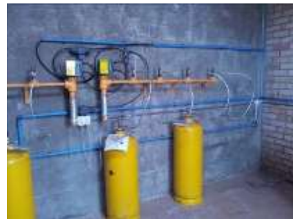
Chlorine room has no scale
