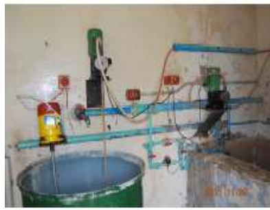
Untidy dosing room with redundant pumps and pipes
