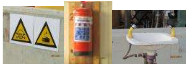
Safety signs and equipment at Mmabatho WTW
