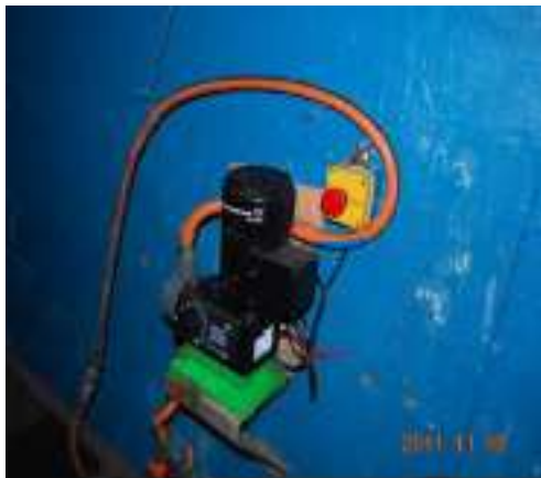
Loose wires and temporary pipes in dosing room
