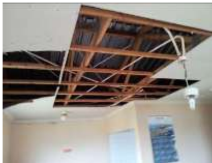
Broken roof in Process controllers change room
