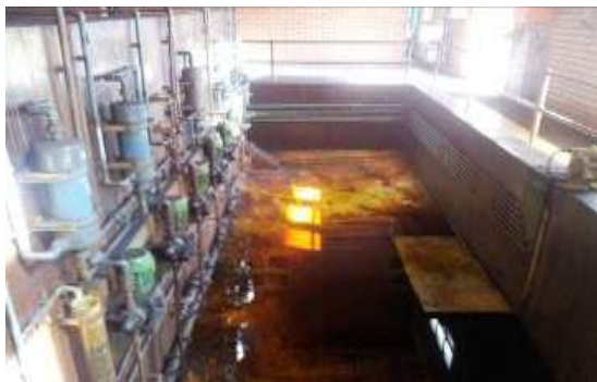
Ferric Chloride dosing area required attention
