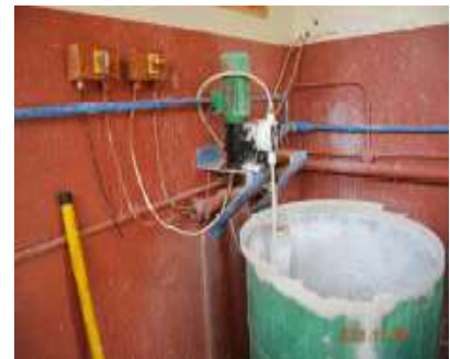
Chlorine dosing room required cleaning
