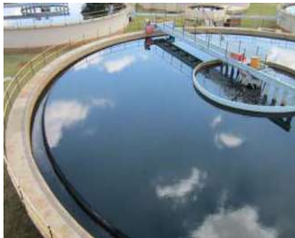
Clarifier with moving bridge
