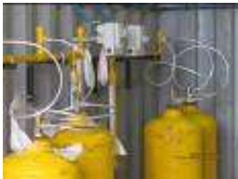
Spare chlorine cylinders in place with level indicator
