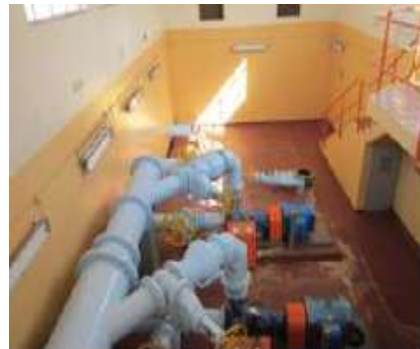
Neat pump station
