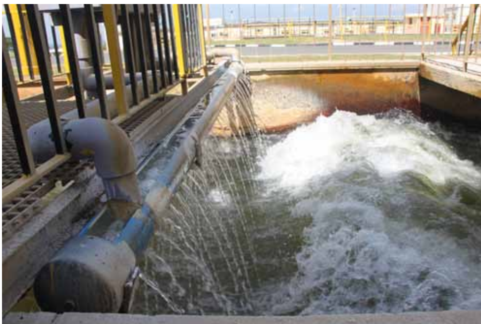
Figure 2: Dosing process at Ethekwini Treatment
